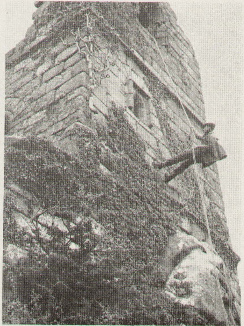
J/Sig Grey descends from an ancient hermit's hut, a height of 100ft.
