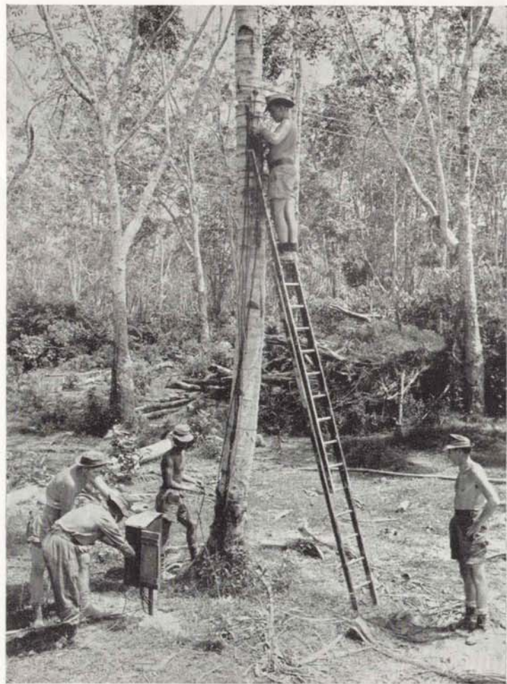
Australian Signals and Royal Signals combine to build a line in the Malayan Jungle.
