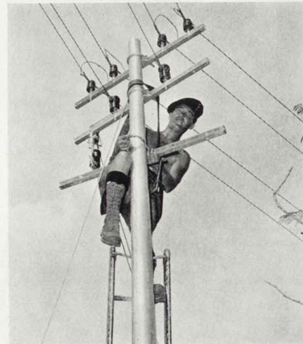
A Lineman repairs an overhead route in the Tropical heat of Singapore.
